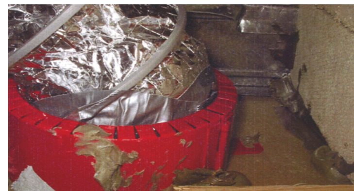
Incorrect use of an intumescent pipe collar on a PVC duct
