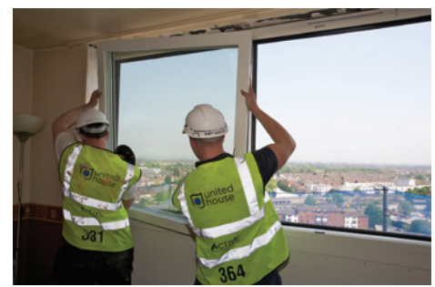
Triple glazed windows with low emissivity coating being installed. The low emissivity glass transmits solar light but not solar heat. (image supplied by United House)
