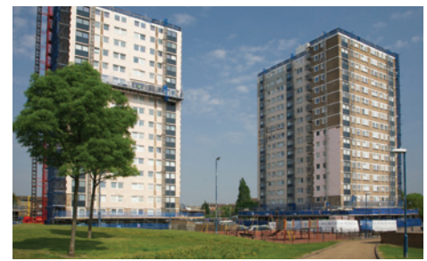
External cladding being applied as part of the combined climate change adaptation and Decent Homes works to the Colne and Mersea blocks in the London Borough of Barking and Dagenham. (image supplied by United House)
