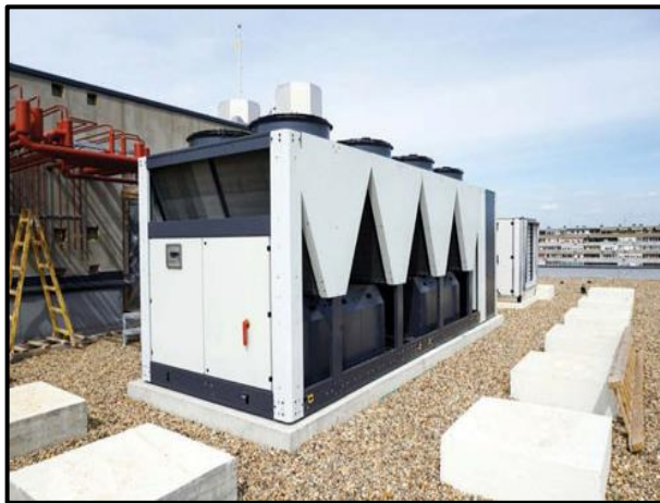
Air-cooled chiller system
