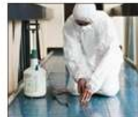
Spray at low pressure; high-pressure spray could disturb fibres from asbestos paper under these tiles
