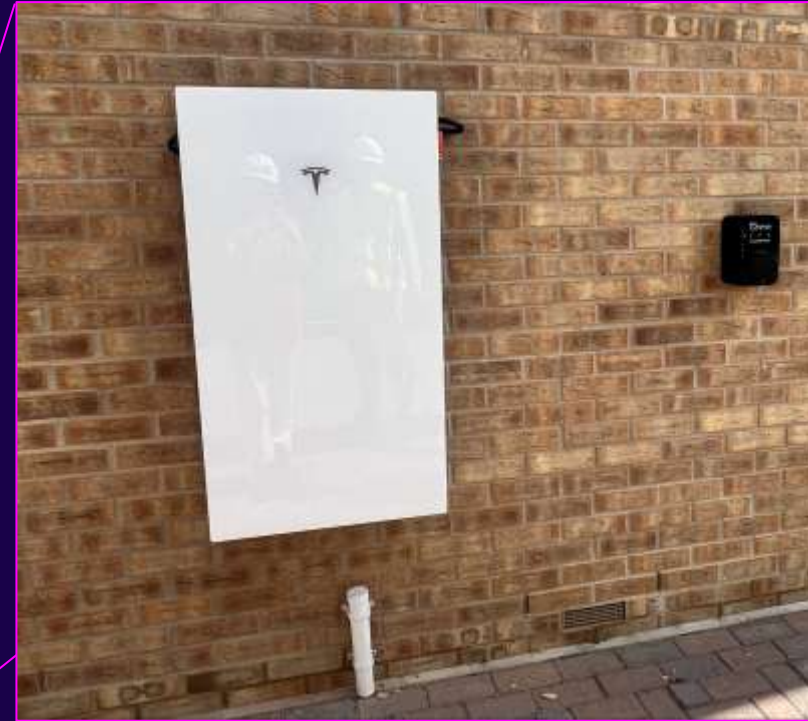
Home Battery (Tesla Powerwall 3)
