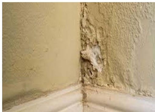
Damp walls causing degraded plaster
