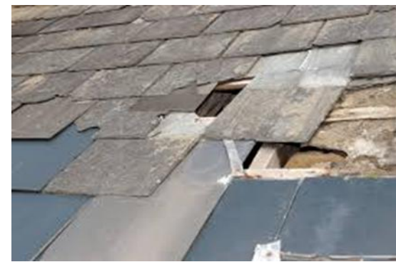
Slipped roof tiles
